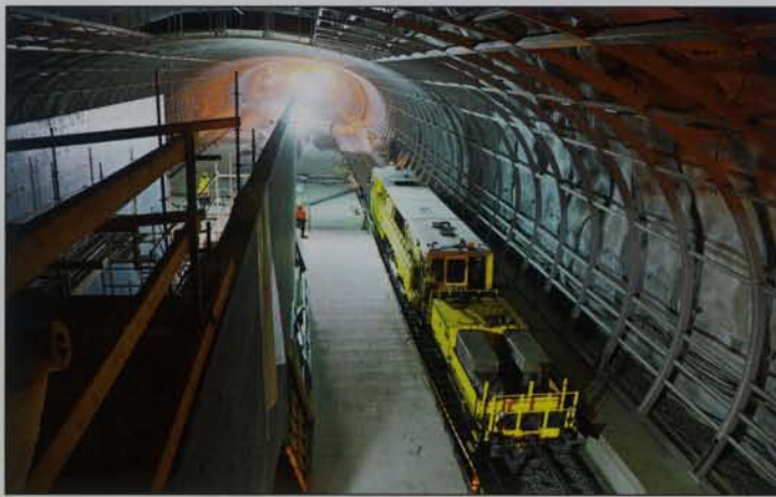
On 19 January 2015 construction was in progress at Lentoasema. The double track is in place, and so is the 230 m long island platform, of sufficient length to accommodate three Class Sm5 EMUs running in multiple. The structure in the left foreground is the housing for the 72 m long escalators, which rise to the surface 45 m higher than the tracks.
