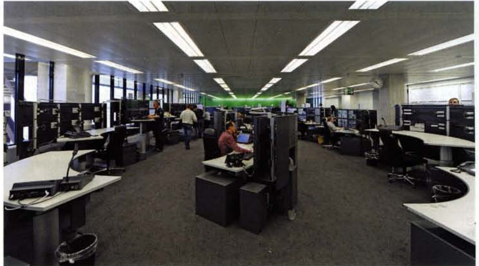
One of the two control rooms; setting up the work-places (in the foreground) (photo: J. Lüthard).
